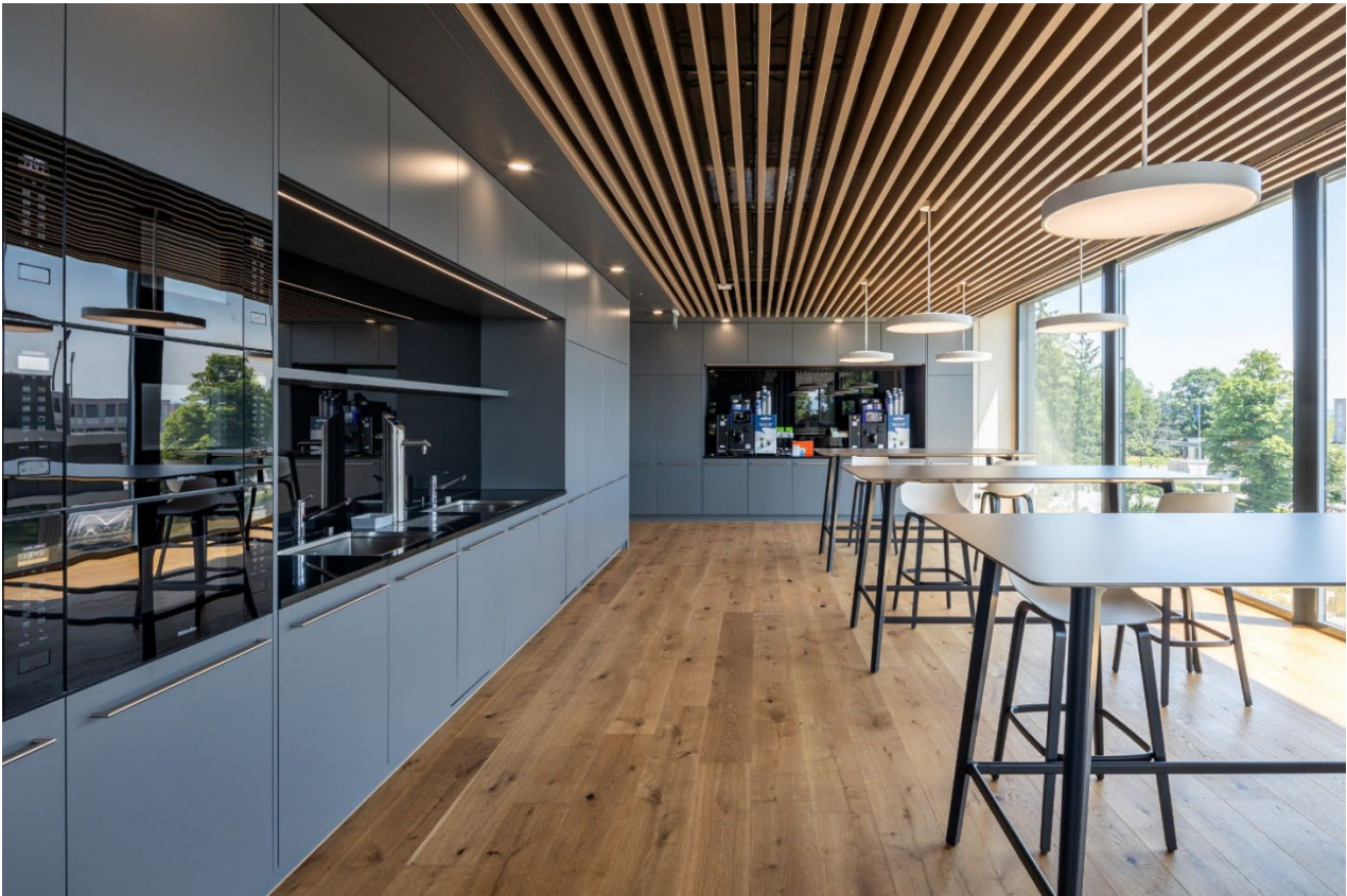
Fig. 10: Baffles constitute a suitable shape for ceiling absorbers. The image shows heating/cooling baffles with an additional layer of sound absorption material (acoustic fleece and mineral wool mats).
